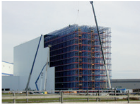
Automated Storage and Retrieval System (AS/RS) rack-supported structure under construction. Source: barroneq.com.
